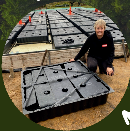
Offcuts placed under the void for recovery & recycling at the end of life
